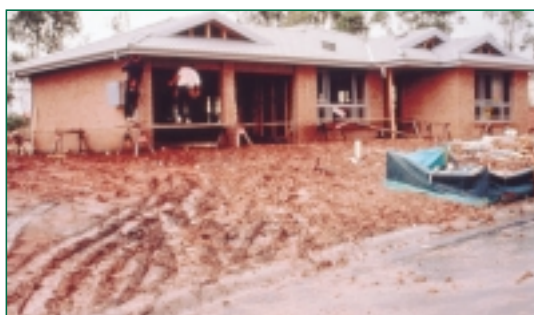
Rain, hail or shine, sediment controls should be in place at all times, prior to, and during building works. This site is clearly causing pollution which flows to creeks via the drains around the site.
