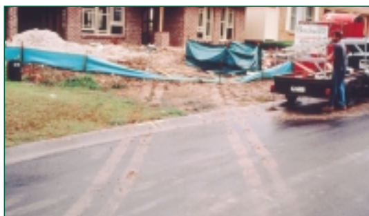
This is a typical situation where a 'entry-exit access' point has not been provided and a tradesman has driven straight over the top of a sediment fence. A stabilised track allows vehicles to enter and exit the site safely during all weather conditions without destroying sediment fences, valuable grass or carrying large amounts of mud and dirt on to the road.
